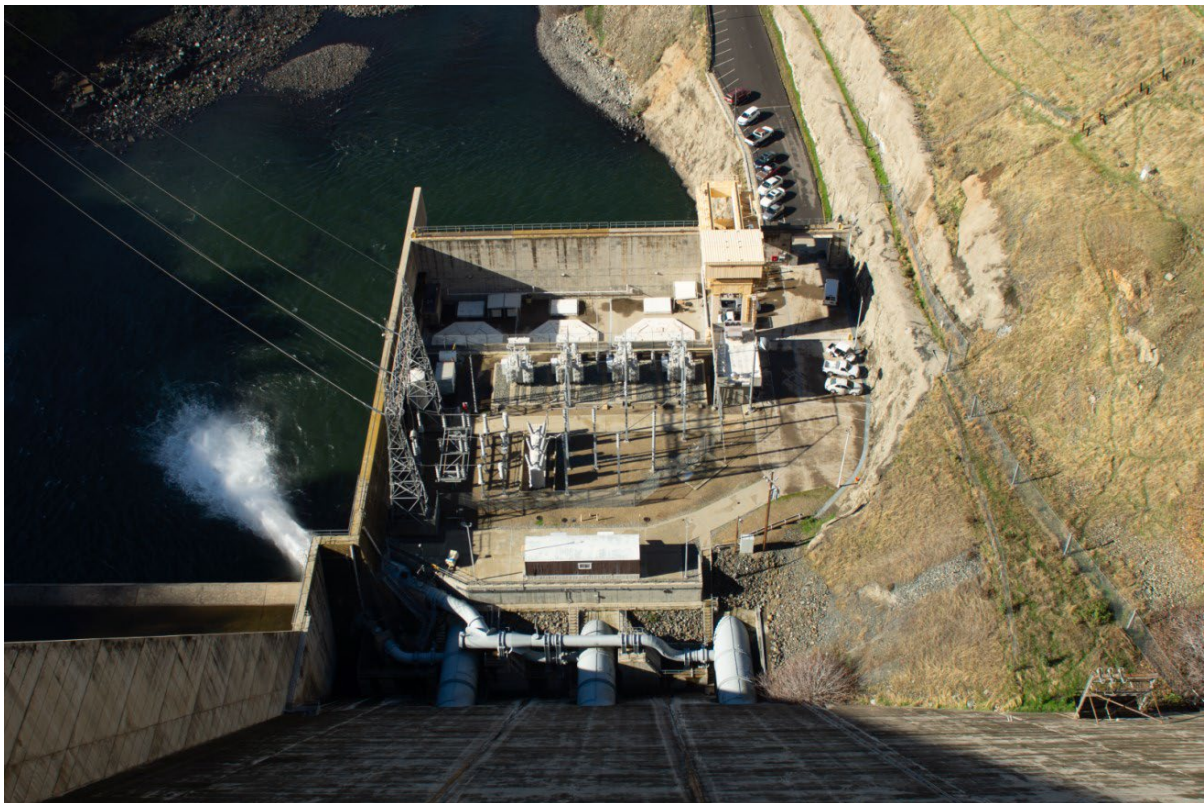
Figure 3. Pine Flats Switchyard and Existing Powerhouse. View from Pine Flats Dam looking West (Downstream)
